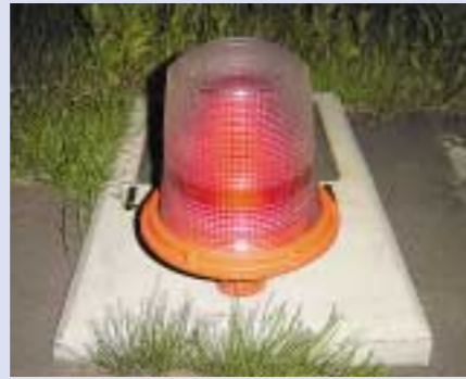
㉑ 過走帯灯 Stopway Light
