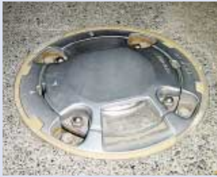
㉒ 停止線灯(埋込型) Stop Bar Light (In-pavement type)
